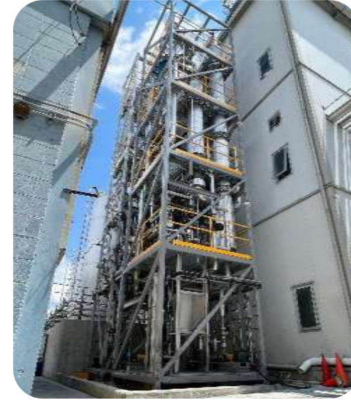
Process water distillation & separation column
