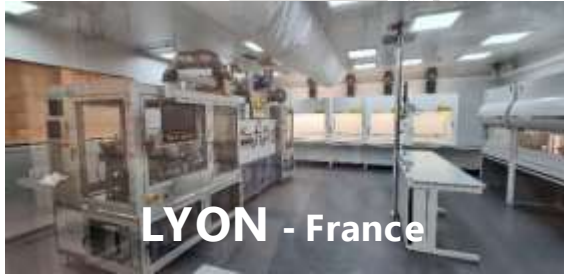
CHRISTIAN COLLETTE EXCELLENCE CENTER FOR BATTERIES
